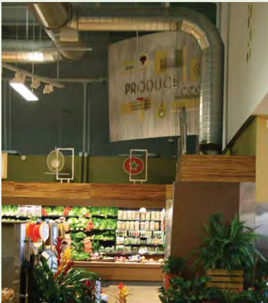
Exposed produce refrigeration ducts efficiently re-circulate the heat, which is then used to warm the building's water systems.
