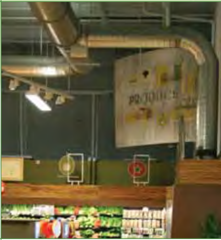
Most of Publix's stores, including its GreenWise store in Boca Raton, FL, include energy-efficient refrigeration and air-conditioning designs.
